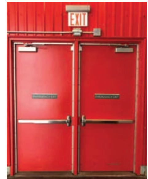
#5077 installed in conjunction with #5077SPB.
