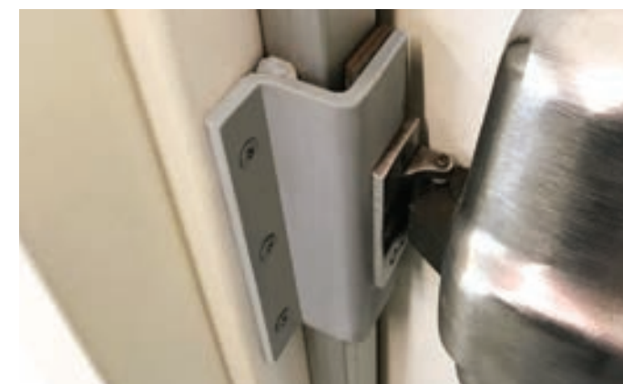
#5077SPB installed at the door strike.
